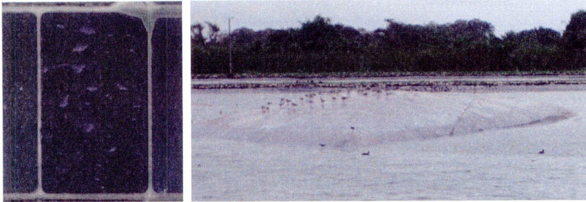
Figure 4-1: Geoliner Failure at Puerto Cortes: A) Satellite View, B) Photographed with Nesting Birds Source: A) Google Earth and B) the Author
